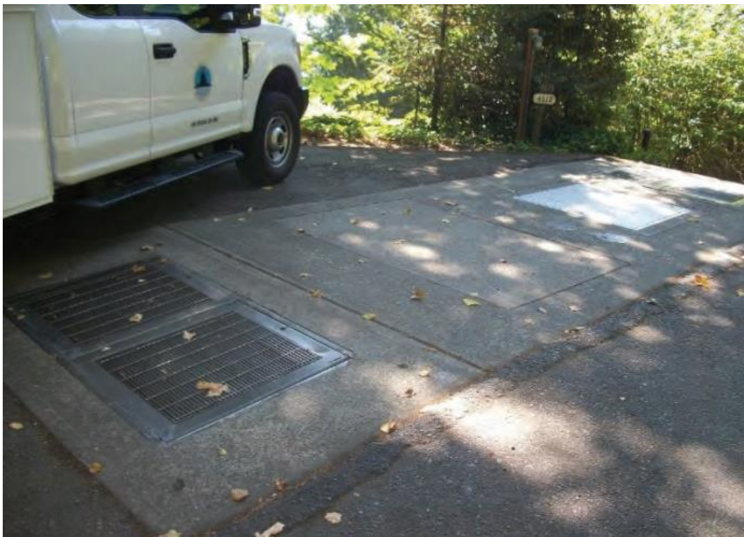
PS 24 – Generator Enclosure
